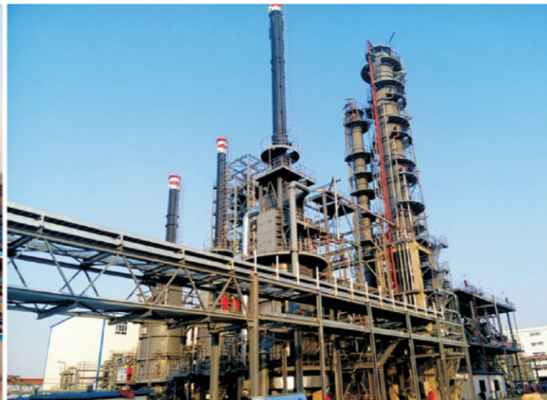
Xinjiang Chaoyuan Chemical 300,000 tons/y White Oil Hydrofining Plant
