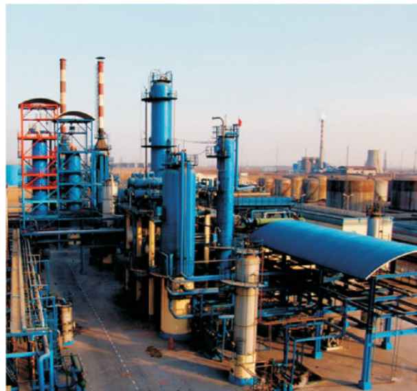
Kenli Petrochemical 1,300,000 tons/y Diesel Oil and Wax Hydrofining Plant
